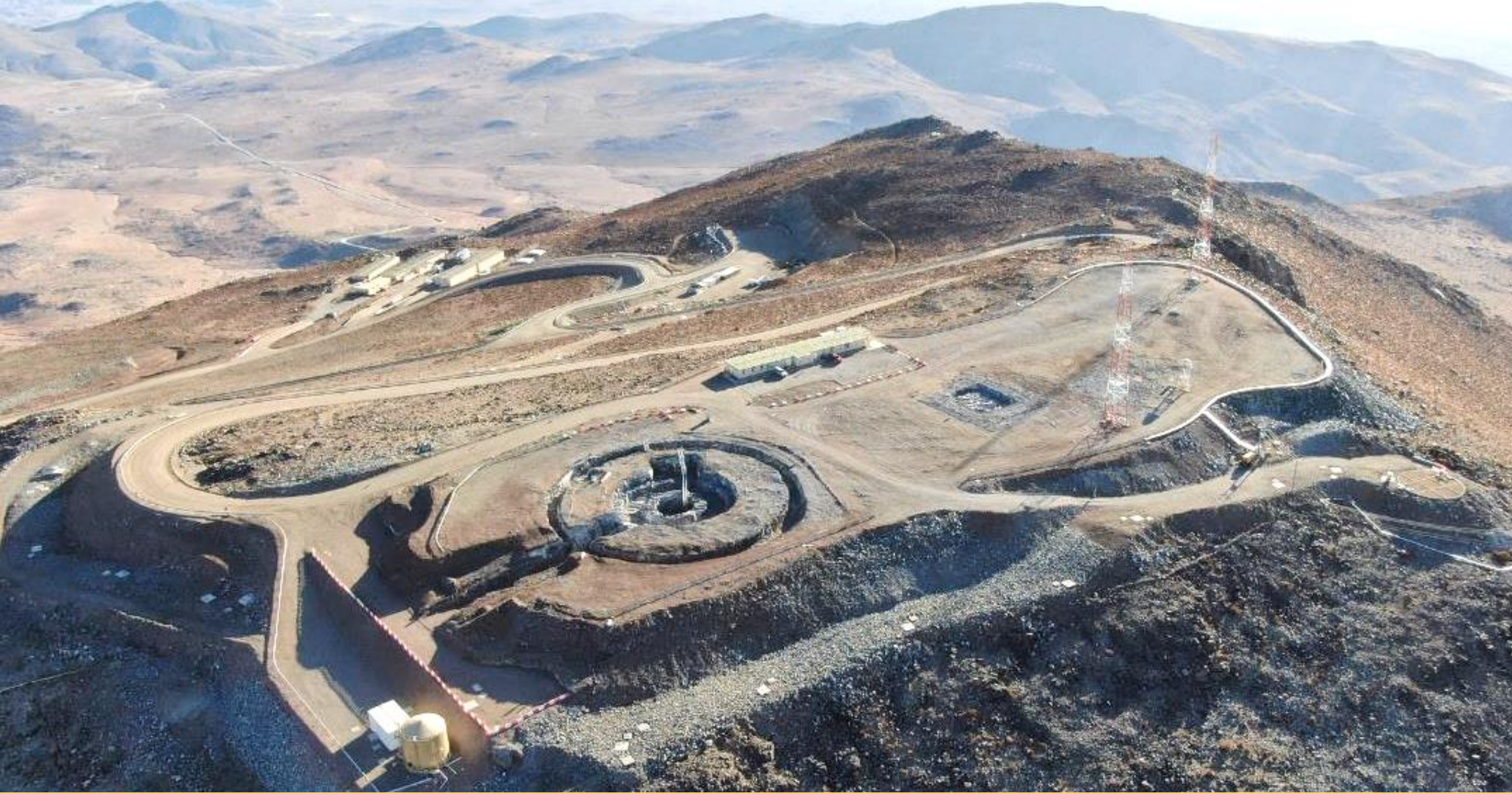
Site : Support facilities are ready to accept telescope and enclosure on site.
